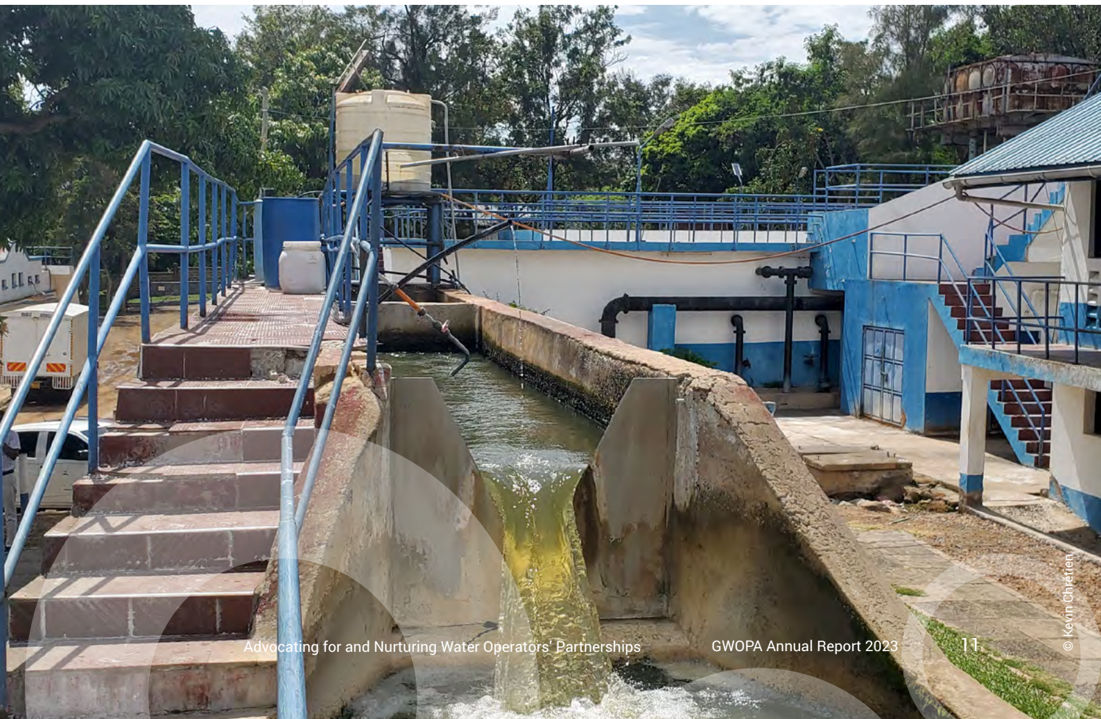
Water treatment plant of EU-WOP partner KIWASCO, Kenya.
