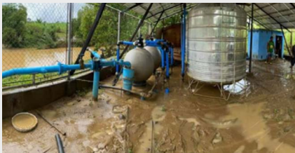
The San Jose-Bugay Water Treatment Facility ceased to operate after being submerged with floodwater © VEI.
