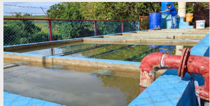
A concrete clarifier was added to improve the treatment design of the facility © VEI.
