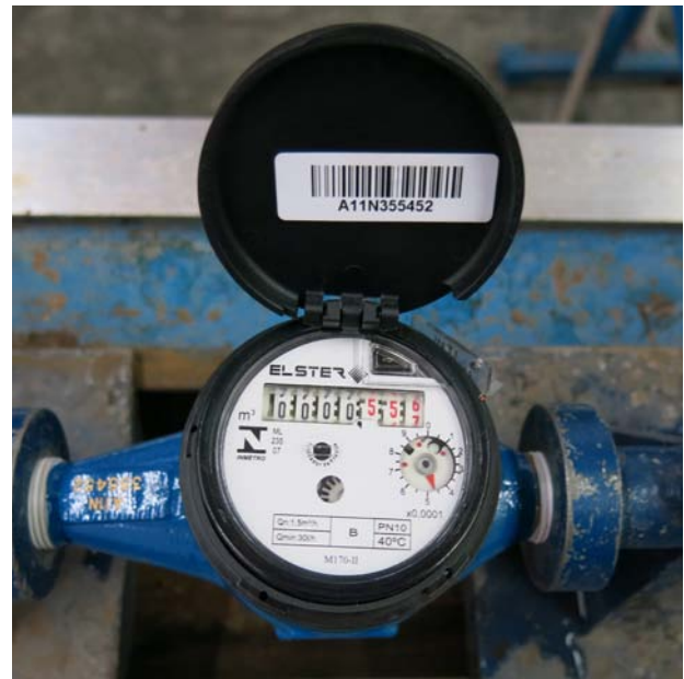
Visit to the Meter Calibration bench at the Alto Molino water supply plant in Salta
